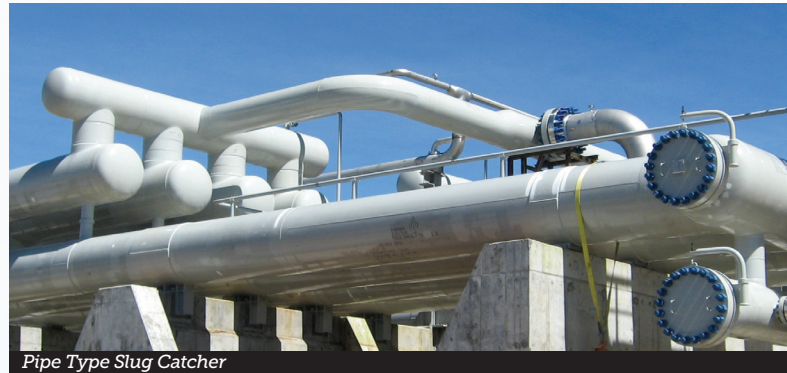
Pipe Type Slug Catcher
